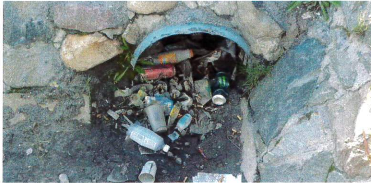
Driveway Culvert Blocked with Debris
